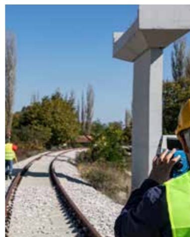
The "Hope" railway between North Macedonia and Bulgaria will be completed with the EU support November 2022
